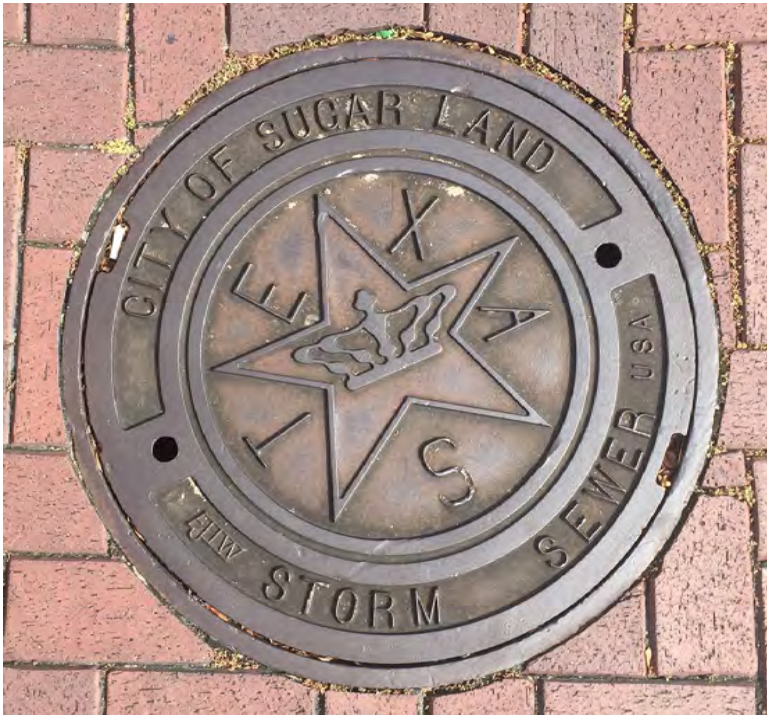
Typical Sugar Land manhole cover.
